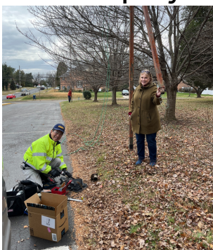
Ken Ow, Jim Short and Diane Walsh-Barberesi repair a parking lot light on a winter afternoon.
